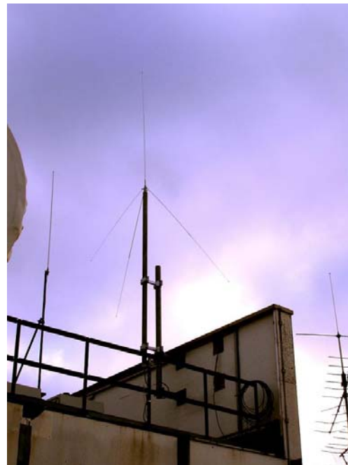
Ground plane antenna
